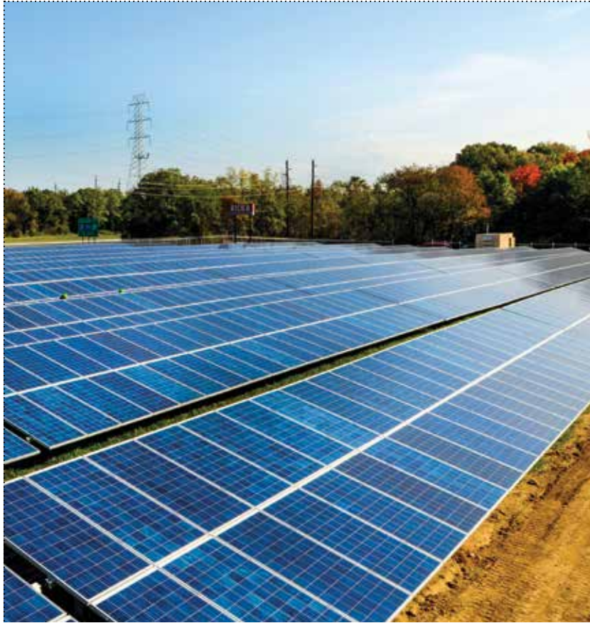
Located in the back of campus near the athletic fields, the 3.2 acre, .74 megawatt solar field provides electricity to dozens of homes, replacing other forms of energy and reducing greenhouse gas emissions.
